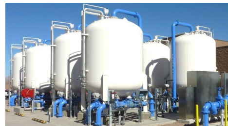
Full-scale conversion of GAC for PFAS Removal at TARP (Tucson, AZ)
