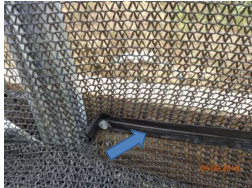
Fabric installation using drip tape and nail or staples to secure the shade cloth
