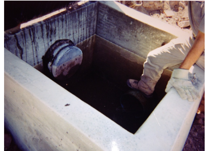
Finished water control structure
