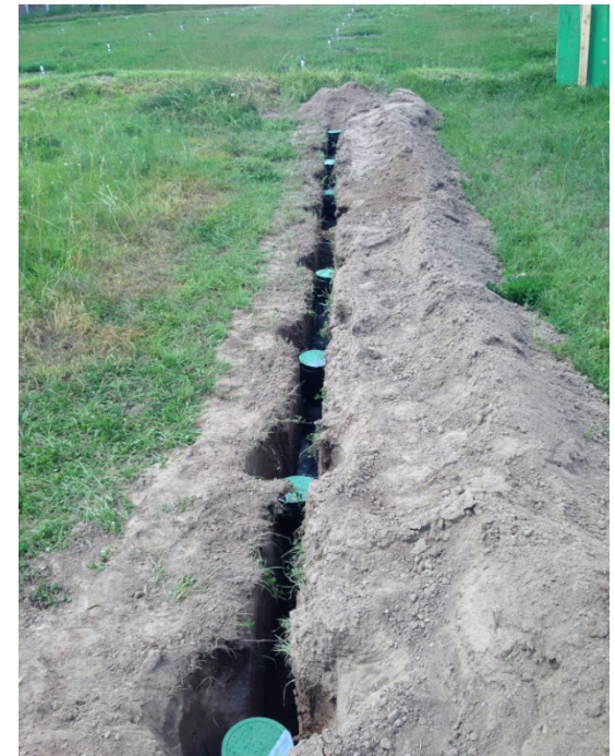
Every row has buried control box
