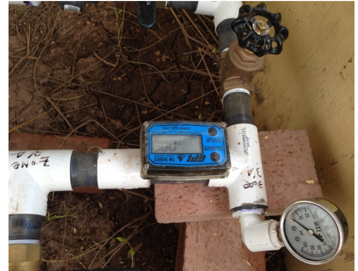
Flow rate meter and valves
