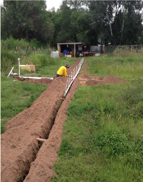
Permanently buried manifold and distribution lines
