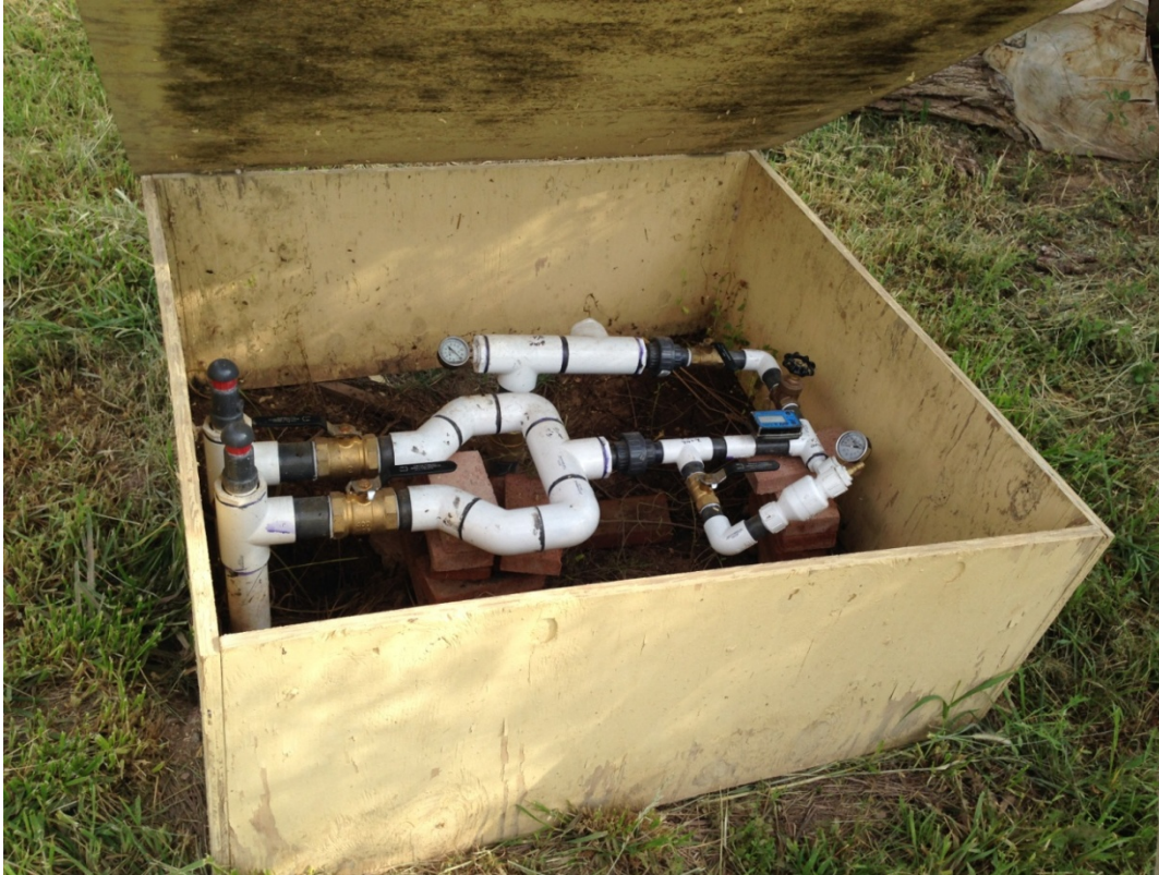
Zone control station directing well water into drip lines
